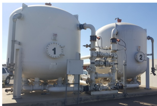
Well Site No. 1 GAC Filters
