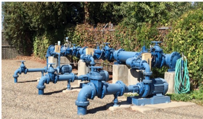
Well Site No. 1 Booster Pump Station
